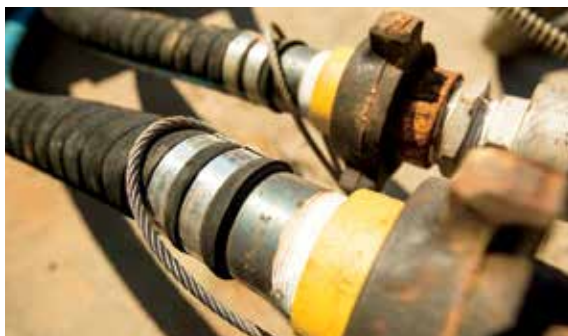
EDF's latest study reveals that methane leaks from some types of facilities are much worse than previously thought.
