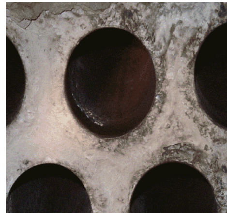
Clean boiler fire tubes
