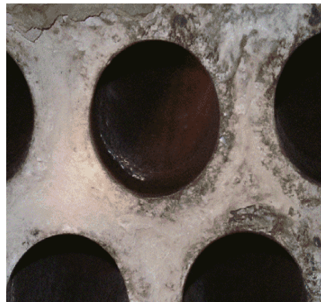
Picture showing clean boiler fire tubes
