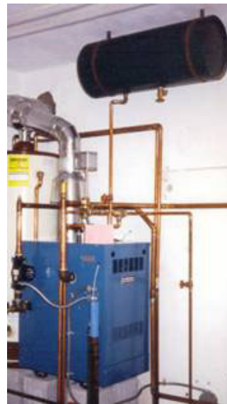
Source: High Performance HVAC
