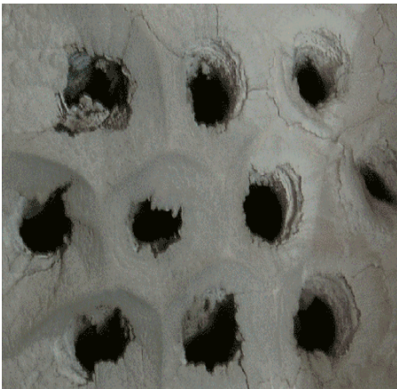
Picture showing dirty boiler fire tubes
